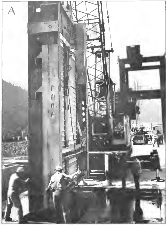
Fish screens are designed to guide fish away from dam turbines. Installing travelling screens at Bonneville Dam (Corps of Engineers)
