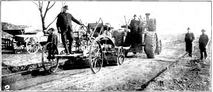
FIG. 2.—PREPARING SET GRADE FOR MACADAM ROAD WITH TRACTION ENGINE AND ROAD MACHINE, ARKANSAS CITY, KANS.
