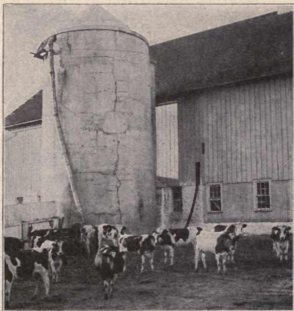
Fig. 9. A solid concrete silo cracked by uneven contraction and expansion caused by extreme cold and extreme heat.
